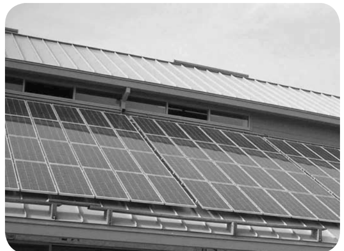
Example of a solar panel
